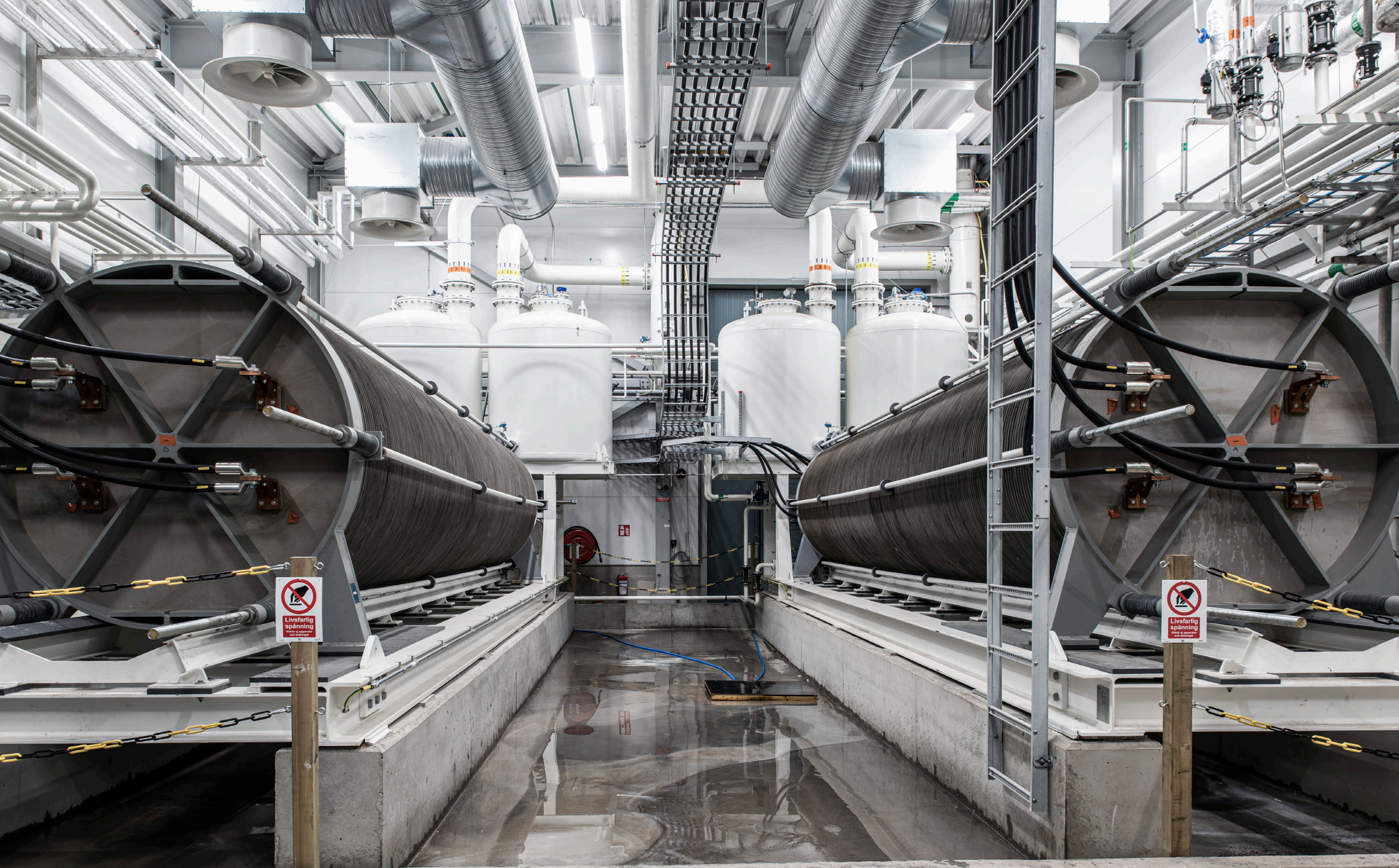
Alkaline electrolyzers produce all the hydrogen used in the direct reduction and hydrogen storage pilot plants.
